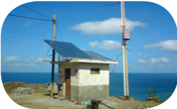
Telecommunication tower powered by PV in remote areas of on the island Sao Nicolau
