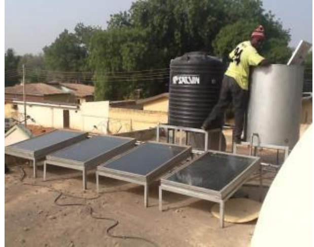
Figure 17: 5.4 m 2 Flat plate collector solar water heating system produce and installed by SERC UDUS at the residence of Dr Aliyu Magatakarda Wamakko at Gawon Nama Sokoto, Nigeria.
