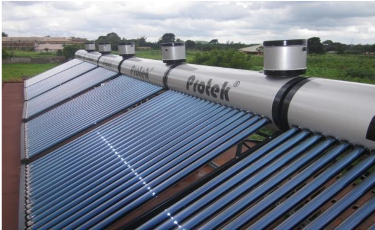
Figure 21: Evacuated tube, thermosyphon systems installed by Dalcy Technology limited at the National Centre for Energy Research and Development, University of Nigeria, Nsukka.
