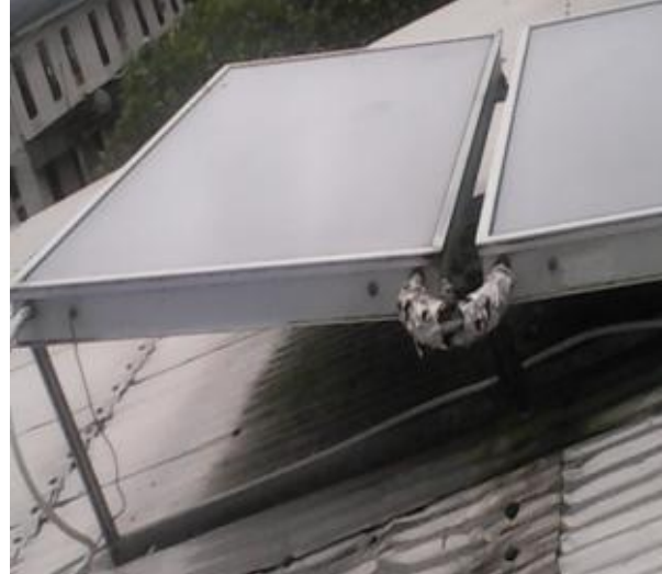
Figure 4: Imported flat plate collector for a pumped system at Port Harcourt.
