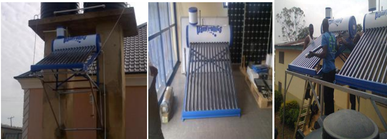
Figure 19: Evacuated tube, thermosyphon systems installed by Pamtronics Nig. Ltd in Jos, Plateau State.
