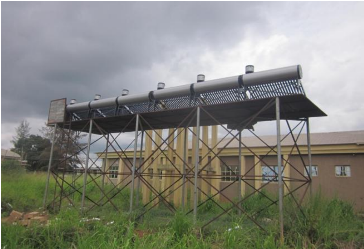
Figure 20: Evacuated tube, thermosyphon systems installed by Dalcy Technology limited at the National Centre for Energy Research and Development, University of Nigeria, Nsukka.
