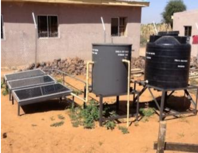
Figure 16: 500 Litres Thermosyphon Solar Water Heater Installed at Danjawa Renewable Energy Model Village(SERC/UDUS)
