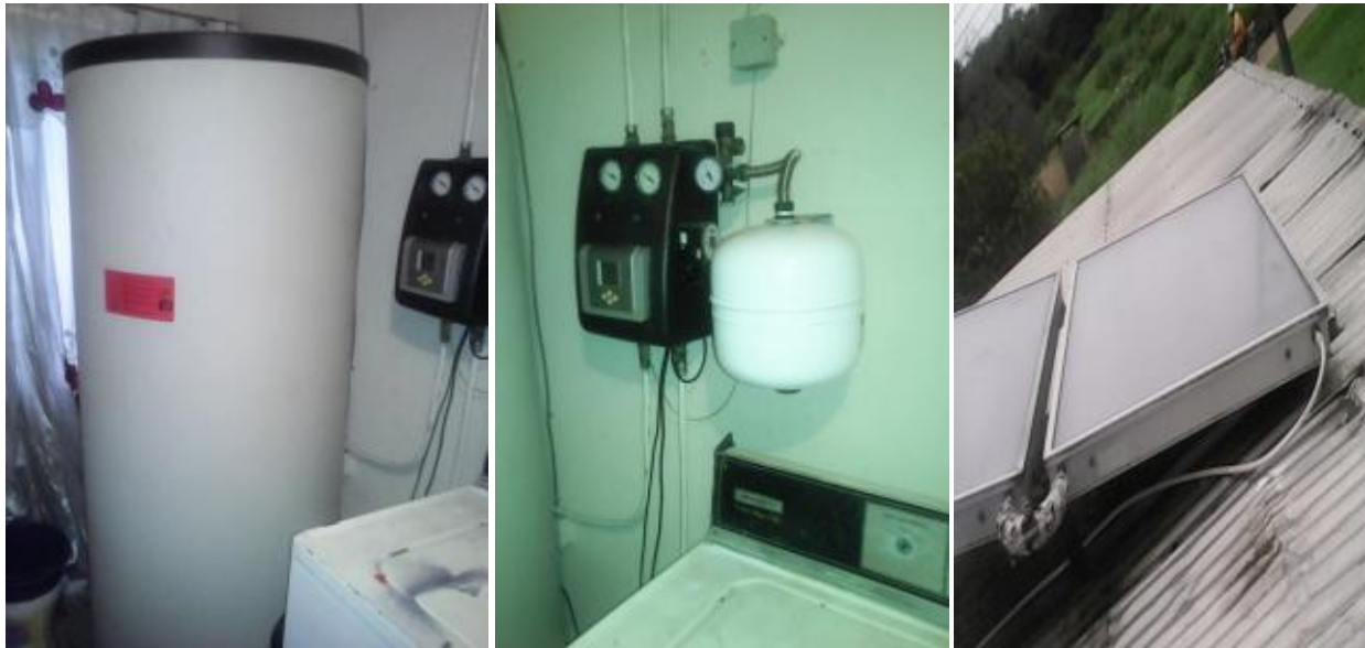
Figure 18: 300 litre, pumped system with 5.016 m 2 collector installed by A. O. Demarg Nig. Ltd. in Port Harcourt, Nigeria.
