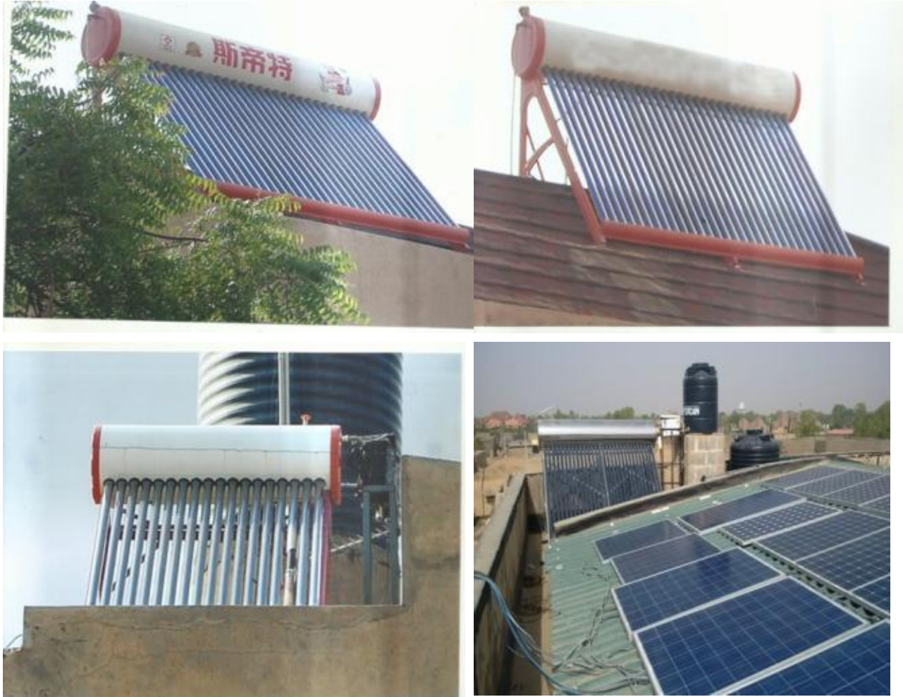
Figure 15: Evacuated tube solar water heating system installed by light Zaman company at Sabon Titi Kano Nigeria
