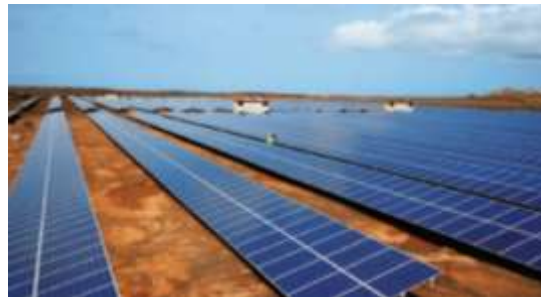
Source: Solar power plant (2,5 MW), Sal island – Cape Verde
