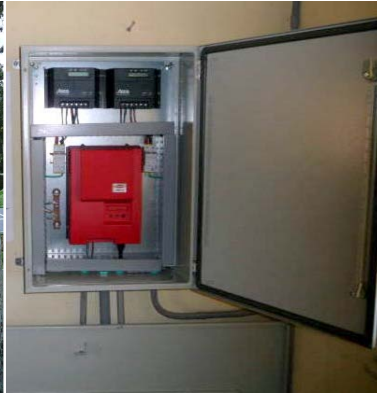
Two charge controllers and inverter per subsystem
