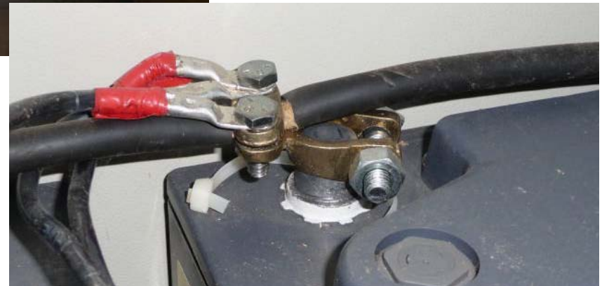
Connections not well tight
