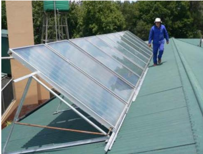
Pumped system at Meerhof School, South Africa
