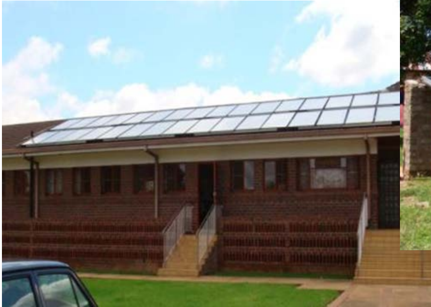
Pumped system - home of retired sisters, Zimbabwe
