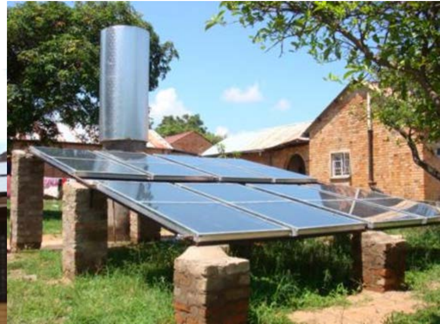
Direct thermosyphon system at Makumbi visitation high school Zimbabwe
