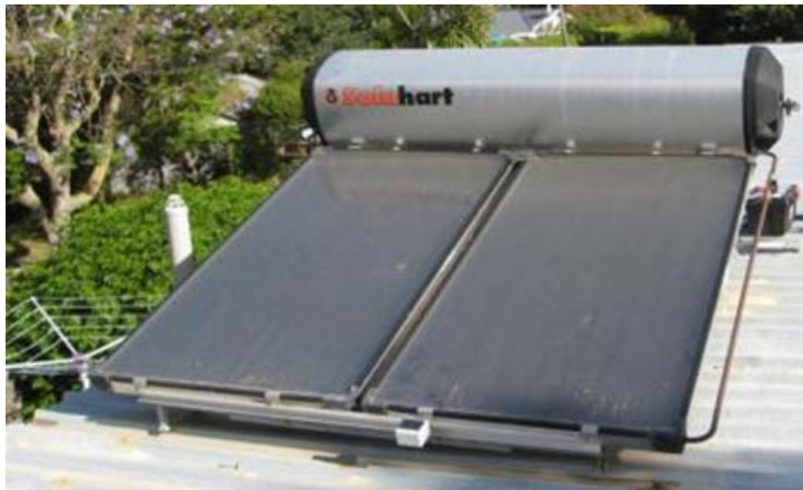
System 1 at a commercial laundry, Cape Town
