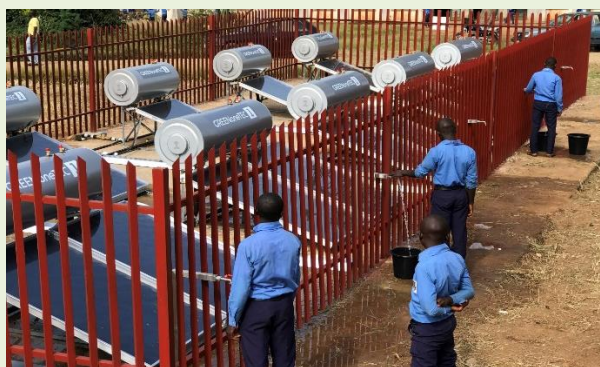
SWH installation at the Government Science Secondary School (GSSS) in Kuru, Nigeria
